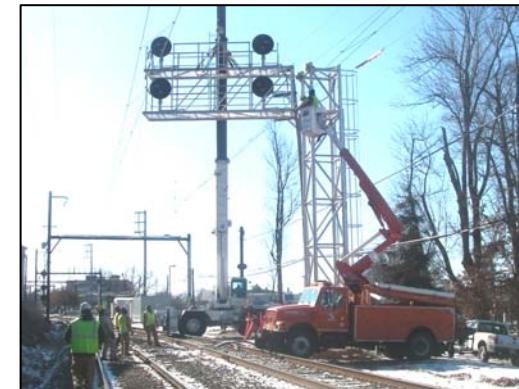
Signal System Modernization Warminster Line
