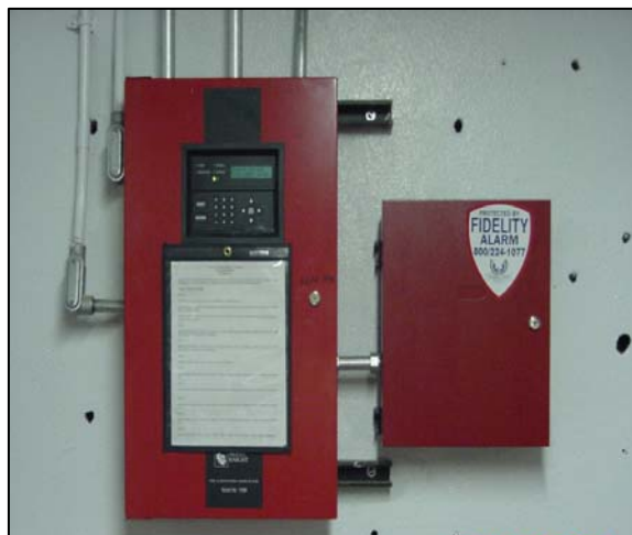
New Fire Detection System
